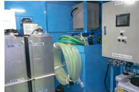
Inside of Aqua Cube (water purification machine room)
